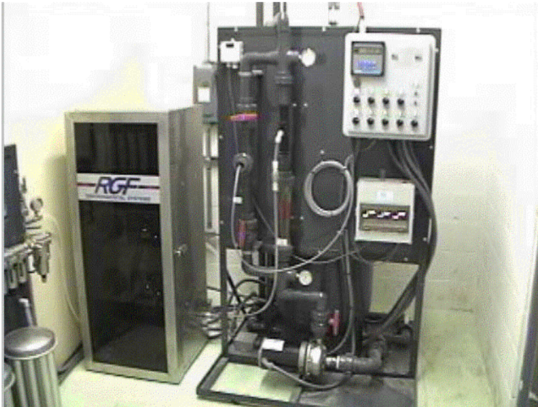
Ozone generator cabinet in left center with control system skid on right. Grey boxes on right of control skid are ozone monitoring and metering devices.
