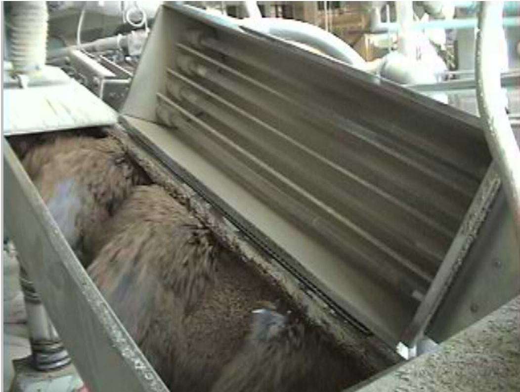
Photo-ionization hood in “off” position mounted over temper bin. Note UV/ozone emitter tubes and grain being rapidly mixed by the auger.
