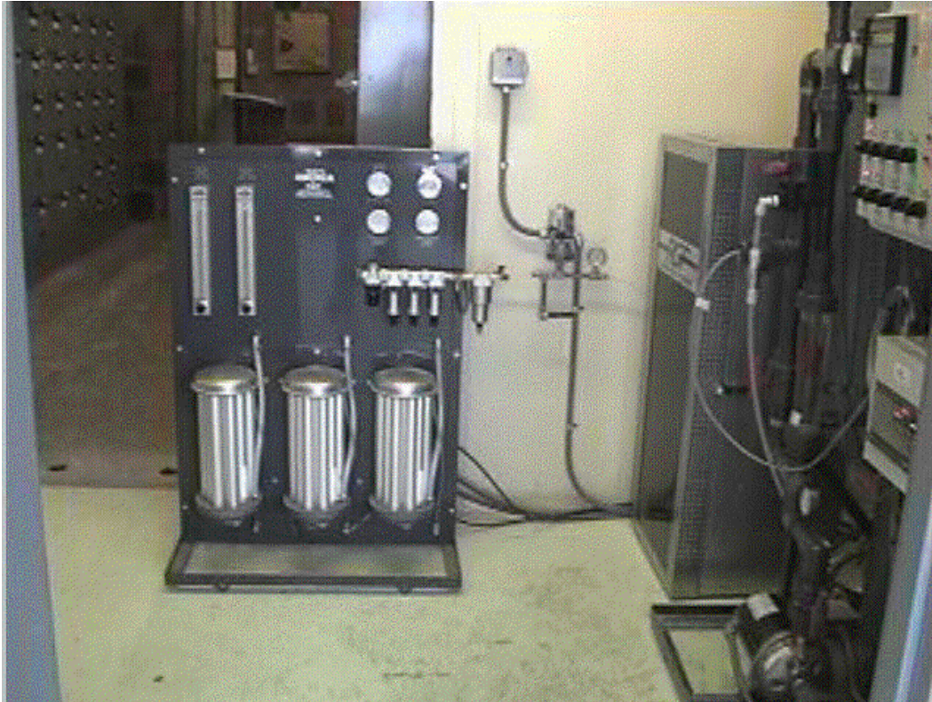
Dry air feed skid supplies 90 percent pure oxygen to ozone generator
